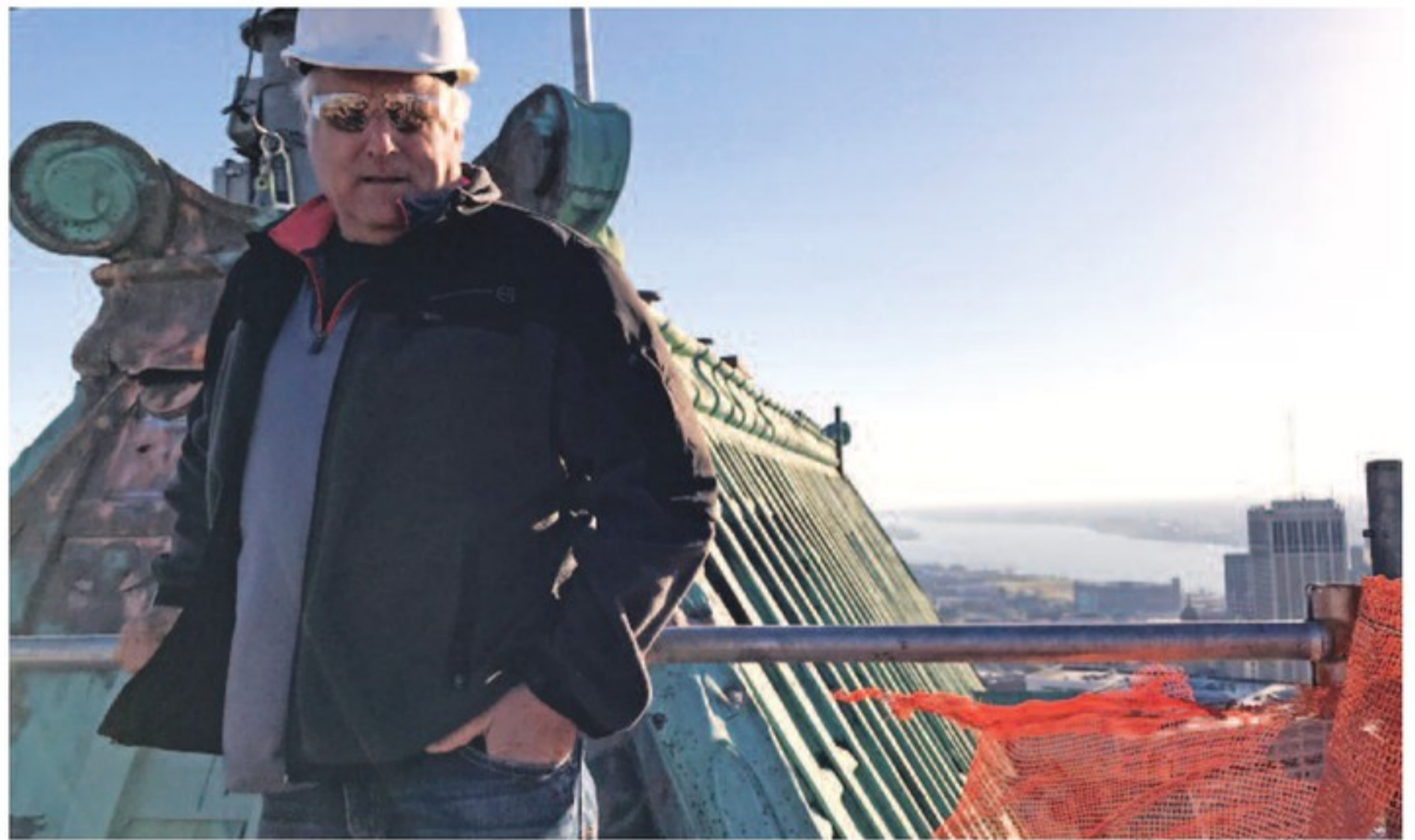
CASS Sheet Metal President Glenn Parvin enjoys a bird's-eye view of Detroit from the top of the Book Tower. Parvin and the entire CASS Sheet Metal team brought the detailed eyes and skilled hands of their collective craftsmanship to the restoration of this remarkable building.
