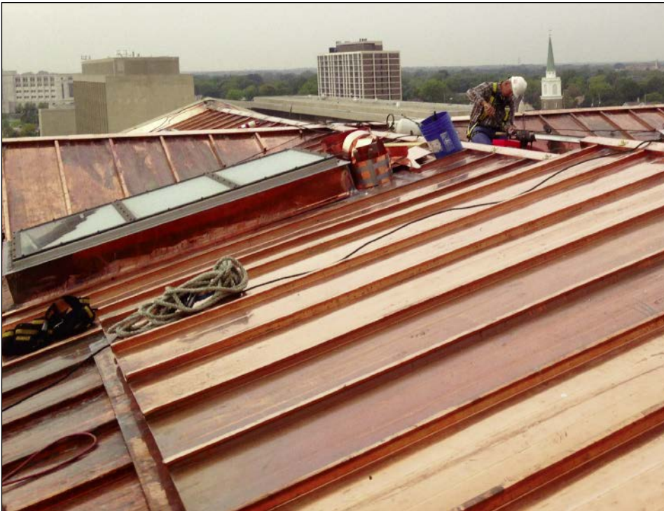
The craftsmen of CASS Sheet Metal are busy at what they do best: Paying meticulous attention to every roofing detail, a work ethic of special importance when working on a national historic landmark that serves as Michigan's official seat of government.
