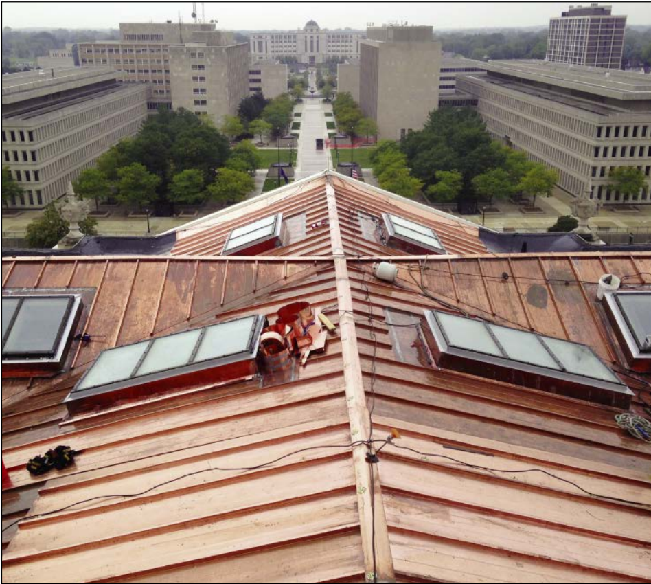
In replacing and installing the Capitol's copper roof, CASS Sheet Metal followed the recommendations of the well-regarded technical manuals: the SMACNA Architectural Sheet Metal Manual and a manufacturer's publication called Revere's Copper and Common Sense .
