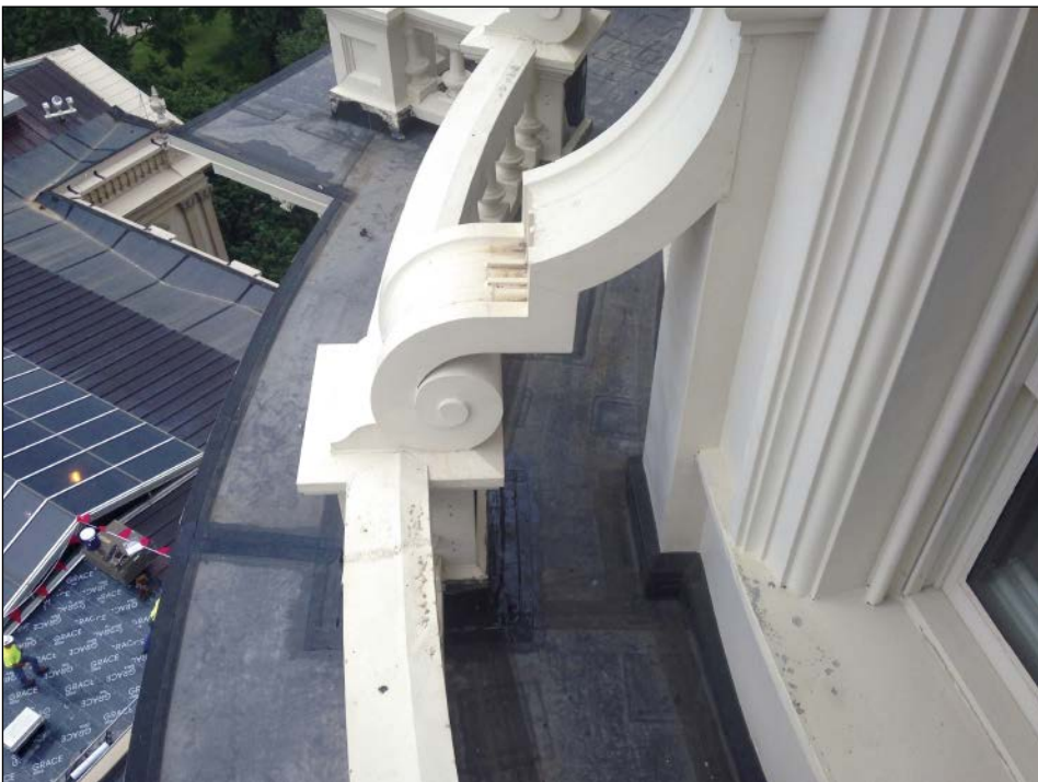
Elegance restored: CASS and Bloom replaced the lead pan roofs on two flat levels of the Capitol dome's drum with a 90 mil Firestone EPDM fully adhered rubber roofing system with 90 mil flashings.
